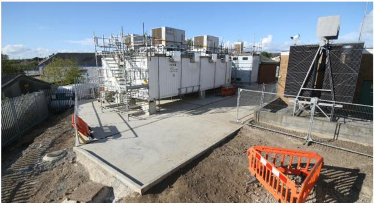
Figure 2 - Rise Carr 2.5MVA batteries and inverters
