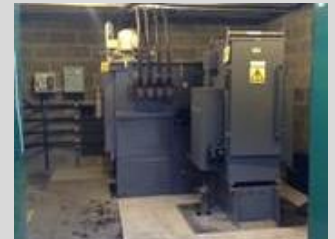
Enhanced automatic voltage control
