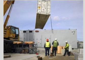
Electrical energy storage
