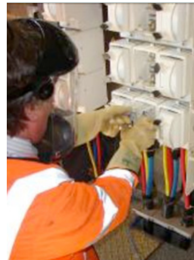
Installation of Kelvatek Bidoyng smart fuses and data gateway hubs. For more photos of the installation visit the project website.
