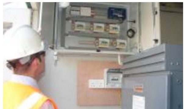
Commissioned Nortech Envoy substation monitoring device. For more photos of the installation visit the project website.
