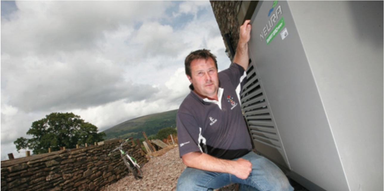
Air source heat pumps have been installed in the off-gas community of Llangattock, Powys
