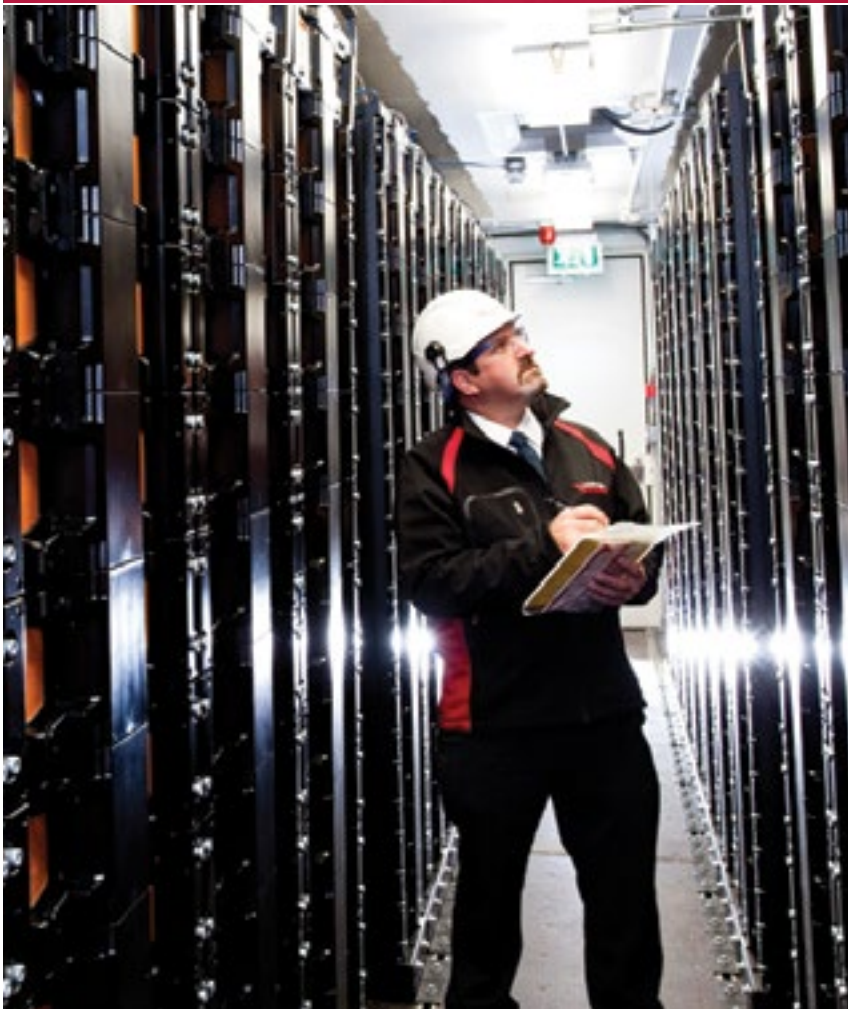
ABOVE: Our 2.5MVA/5MWH energy storage battery at Rise Carr in Darlington.
