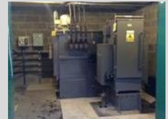
Enhanced automatic voltage control
