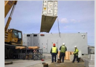
Electrical energy storage
