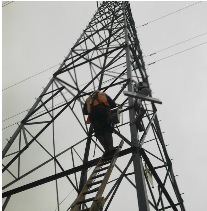
Figure 3 Local Controller installation on tower line
